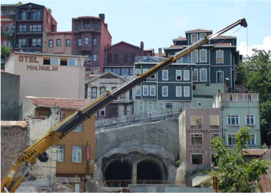
Metro construction in a World Heritage district in Istanbul. (Photo: V. Marquart, 2012)
