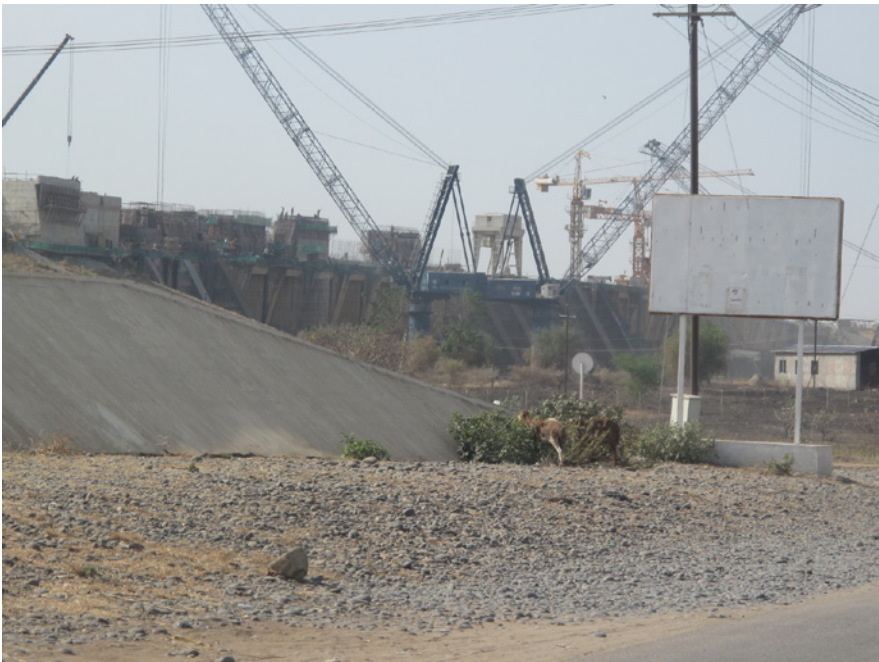
Heightening the dam at Roseiris, Sudan, which will cause the displacement of many farmers. (Photo: G. Schlee, 2009)
